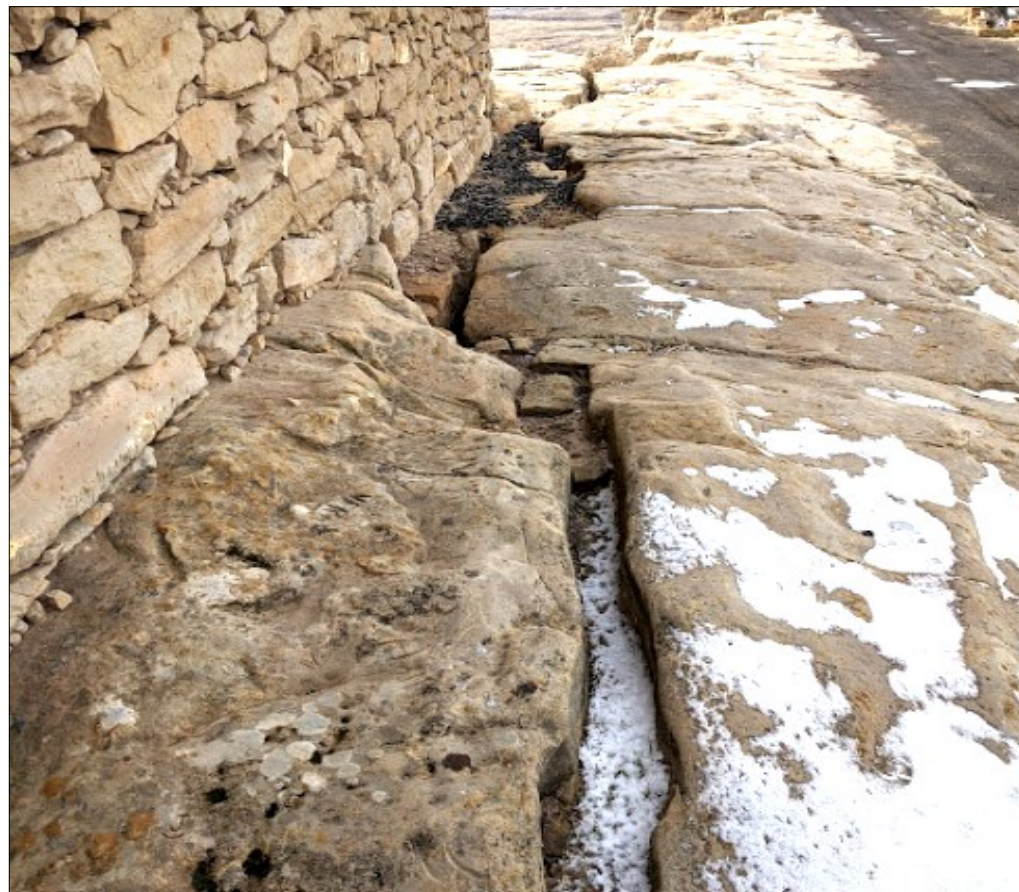
Sightings of more cracks on First Mesa have been reported. Everyone is reminded to be cautious and alert when attending ceremonies and events on the Mesa.
