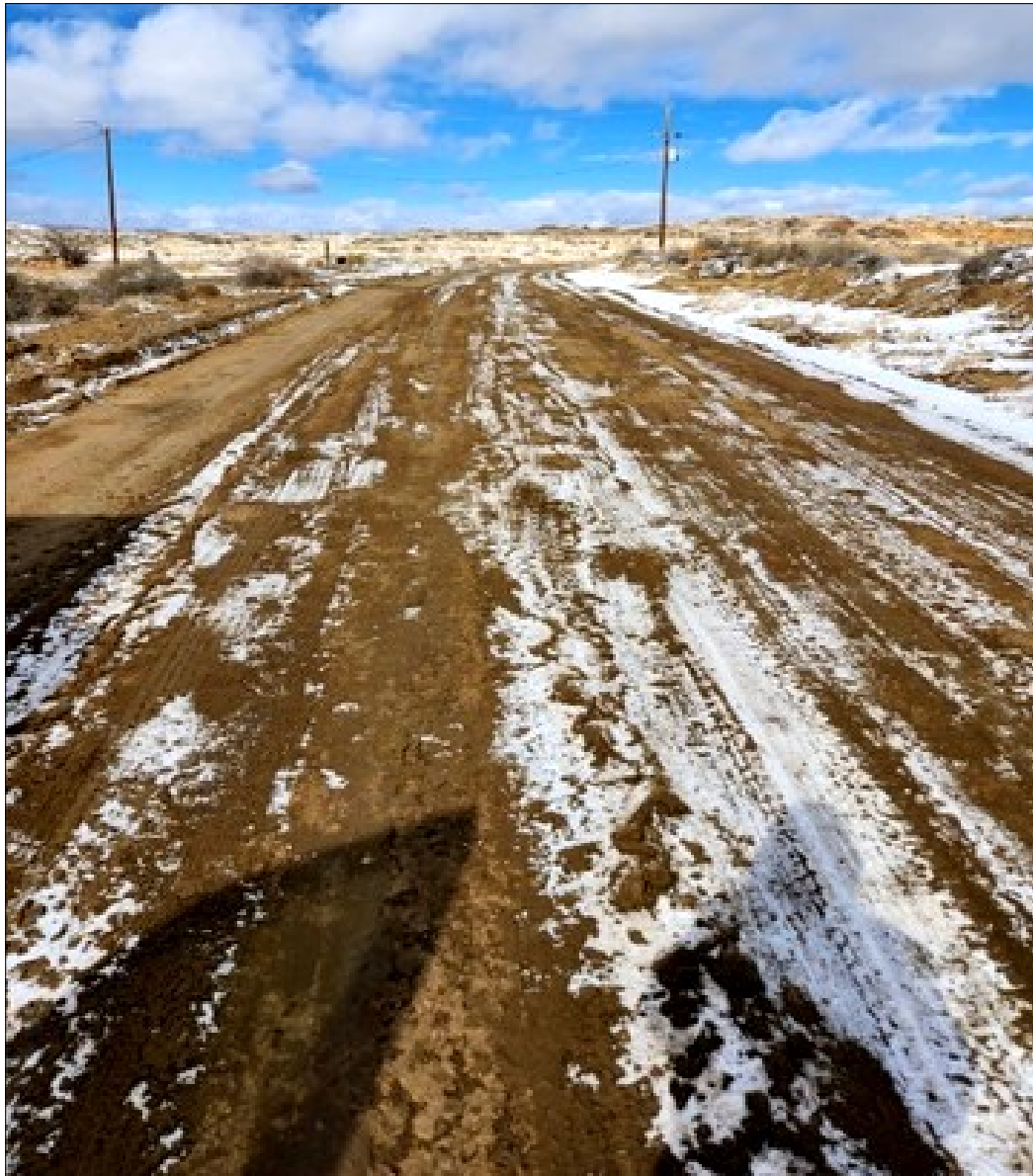
IR10 was plowed making it more passable for local school busses to pick up students from behind the Mesa.
