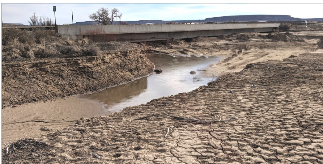
Standing water indicates dense saturation
