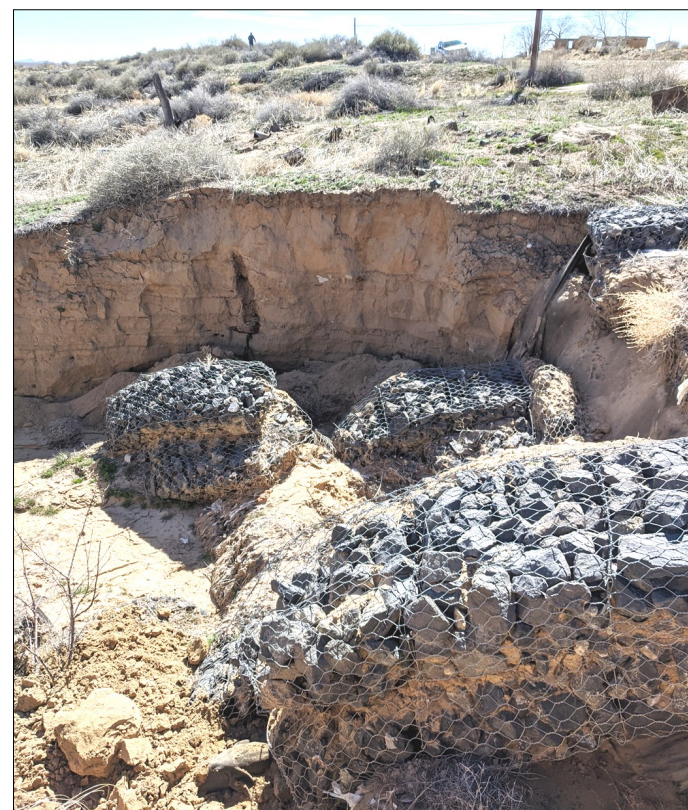
Gabion near Coyote Springs flowing down to Hwy 264 used to catch sediment to slow the flow of water
