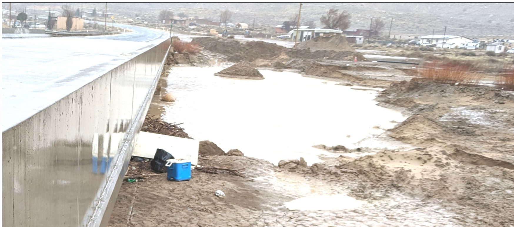
Debris built-up under east Polacca Bridge, after the snow and rains in March
