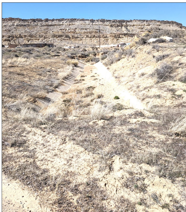
Concrete drainage near old Polacca Day School filled with sediment
