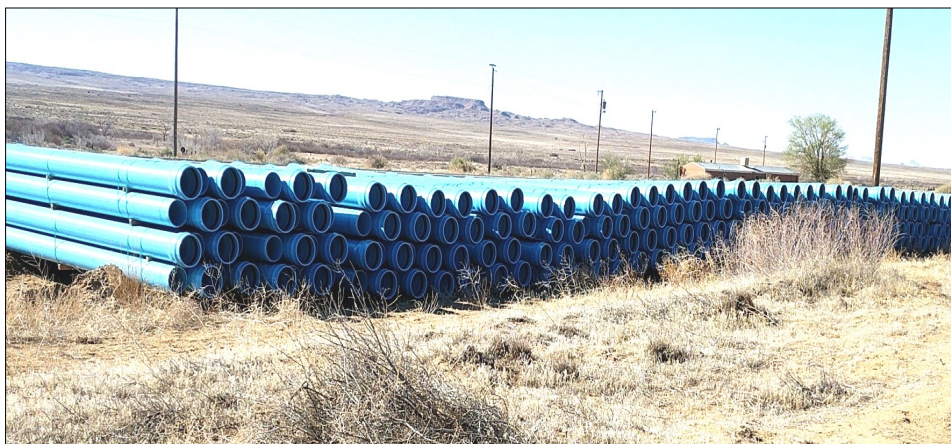
Blue water pipes have been delivered to sites along the water line route
