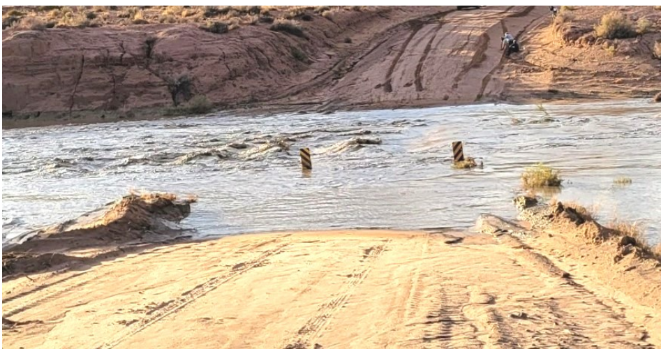
Heavy rains flood bridge at Dinnebito Wash.
