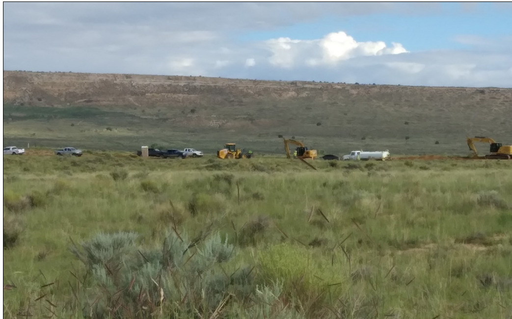
Construction work continues alongside Hwy 264 as pipeline is installed, enroute to Keams Canyon
