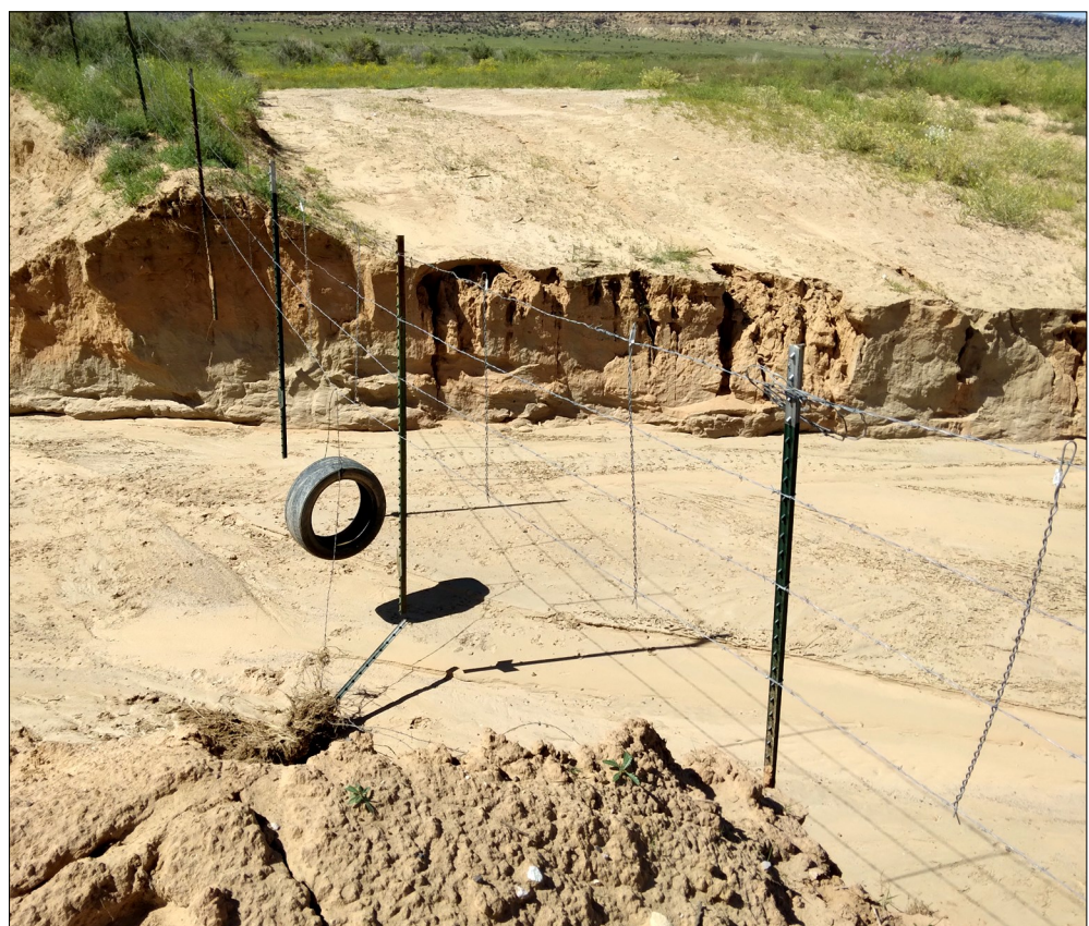
BIA Route H60 (Low Mountain Road) received major damages from the last few rainstorms. This created much hardship for students attending Hopi High School as well as area bus drivers and for emergency services; i.e. ambulance and police.
