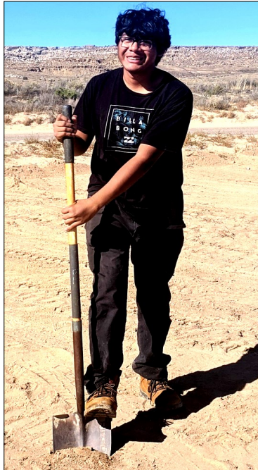
Quintin Nahsonhoya (Skate 264) breaks ground near Tewa Sand Clan ball field on Nov 5. Construction work on the foundation began Nov. 6—Nov. 7. The next step is installation of a Skate ramp donated by Cowtown S.K.A.T.E.
