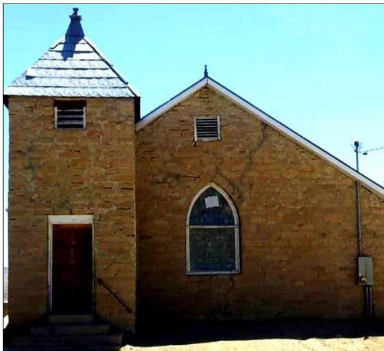
Old sanctuary in early years showing signs of cracks
