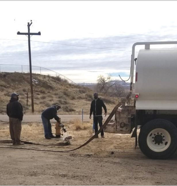
By mutual agreement and partnership, construction workers haul water from the Polacca Water System to Kykotsmovi Village for new business development.
