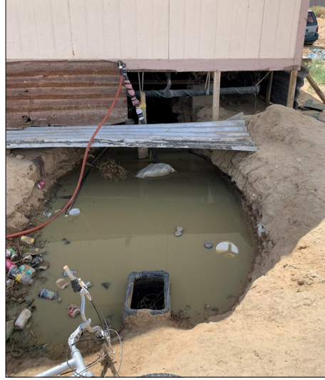
Water Leaks must be corrected immediately homeowners
