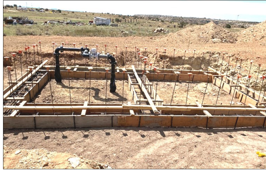
Booster station building and piping for HAMP project
